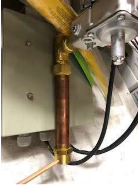
Pointing at the endcap of Condensation Chamber
